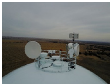
Wireless equipment on the Ravenna water tower.
